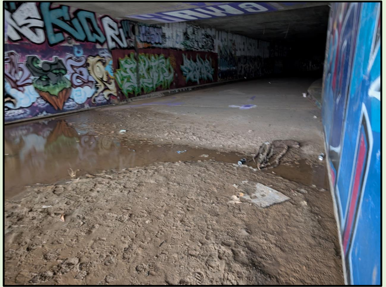
Serrano Creek Tunnel – Note Standing Water and Graffiti
